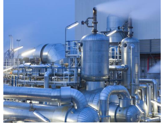
SMR of natural gas to make hydrogen.
